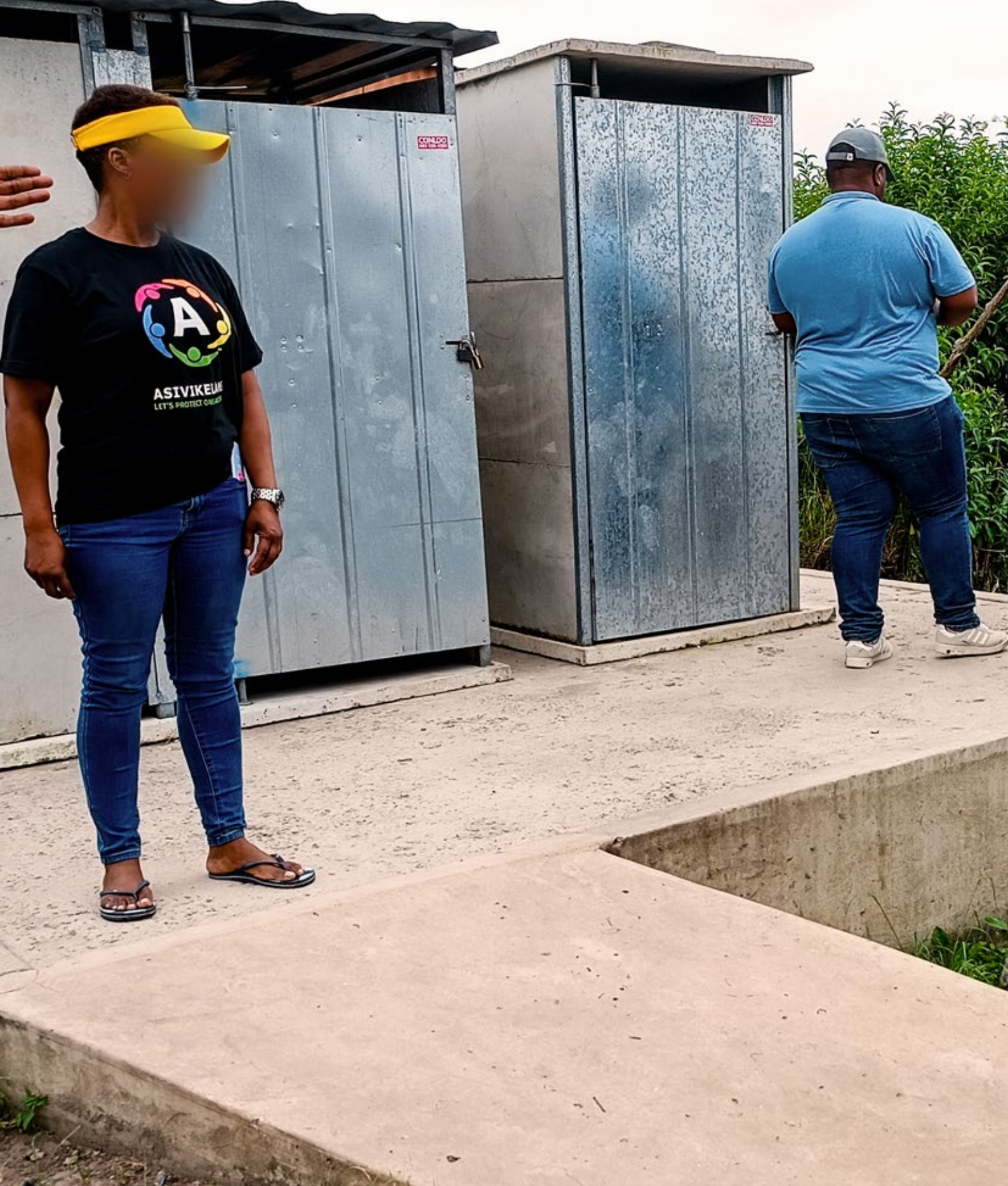
A Communal waterborne flush toilet in the Hani Park informal settlement in Buffalo City in 2024. The toilet has a wheelchair ramp and one of the toilets is suitable for use by persons with disabilities. The toilets can lock from the inside and is well-maintained. There is a basin with a tap, and an additional communal standpipe which is installed with the toilets. Photo Credit: Asivikelane.
