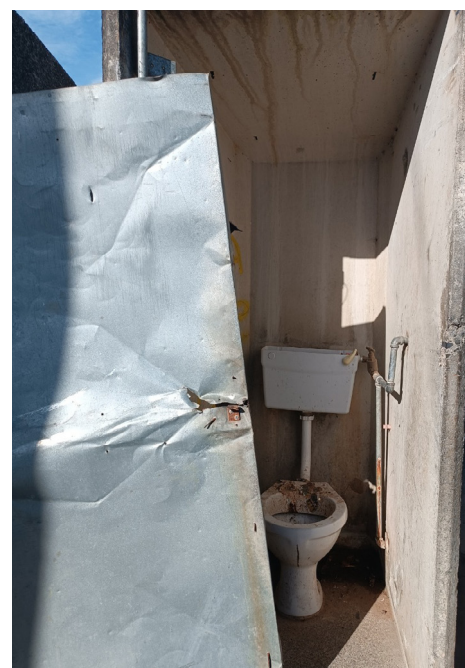
An unusable communal waterborne flush toilet in the Slovo Park informal settlement in Buffalo City in 2024. The door is broken, and the toilet seat is missing – it is dirty and unusable. A lack of repairs and maintenance, and too many households using the same toilets has a massive impact on the useability of a communal flush toilet.
