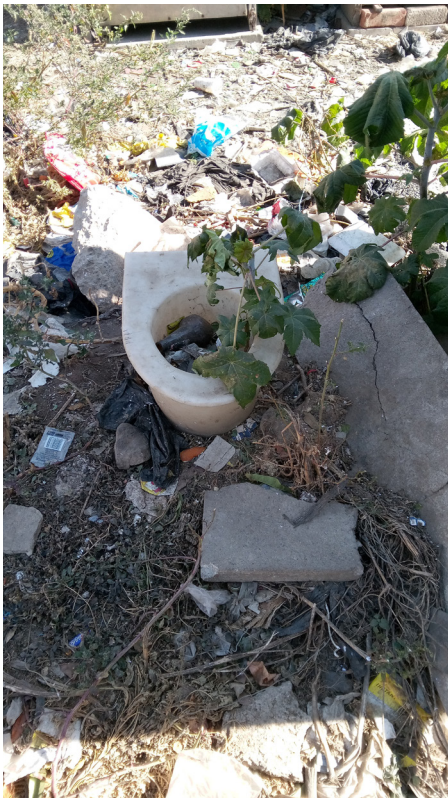
A demolished legacy VIP Toilet in Johannesburg where the pit was not fully decommissioned at the time the picture was taken in 2024. This poses significant health and safety risks.
