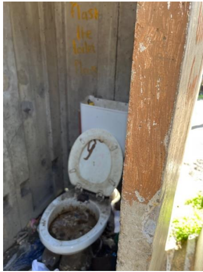
Figure 1 Toilet in Victor Molosi, blocked toilet
