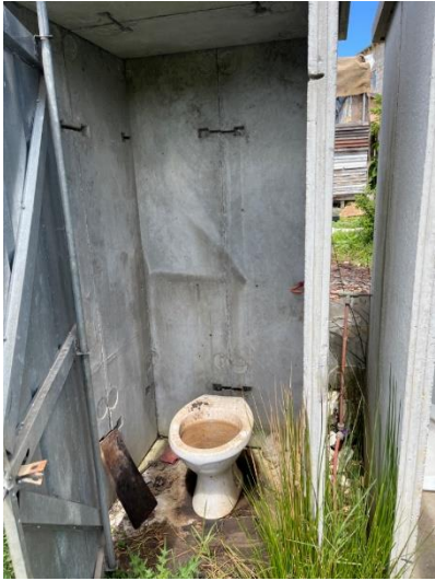
Figure 3 Toilet in Victor Molosi, no flushing system
