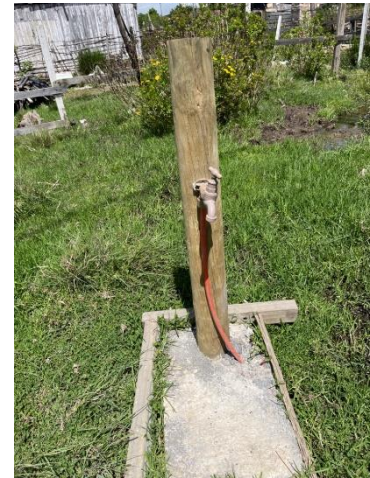
Figure 5 Tap in Rosemore, no water coming out
