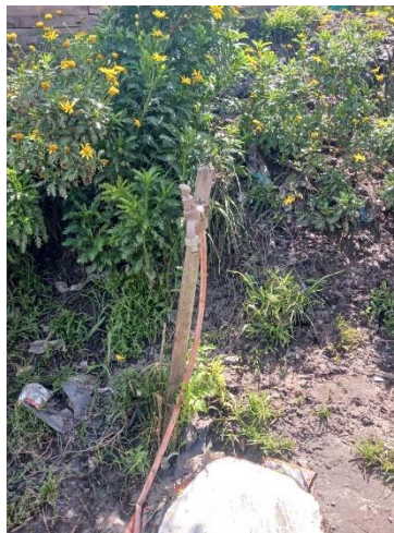
Figure 4 Tap in Rosemore, low water pressure
