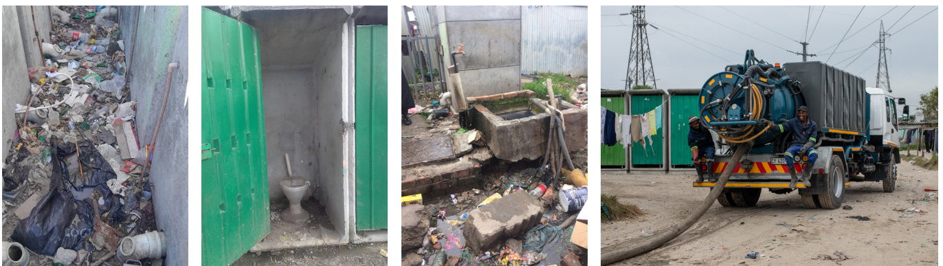
Left to right: Drains blocked (Khayelitsha), broken toilets (Europe), broken taps (Imizamo Yethu), and toilets drained (Khayelitsha)
