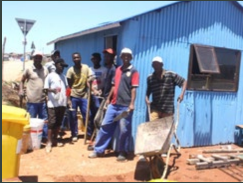
GOOD NEWS Nelson Mandela Bay Concrete slabs built for water tanks, workers employed
