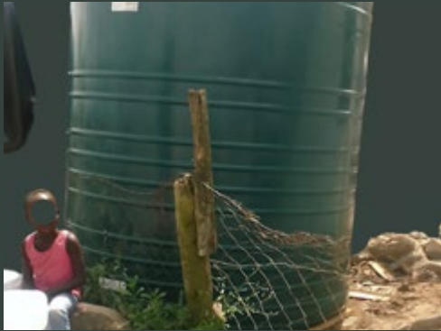
GOOD NEWS Buffalo City Metro 10 new water tanks were installed in Nompumelelo
