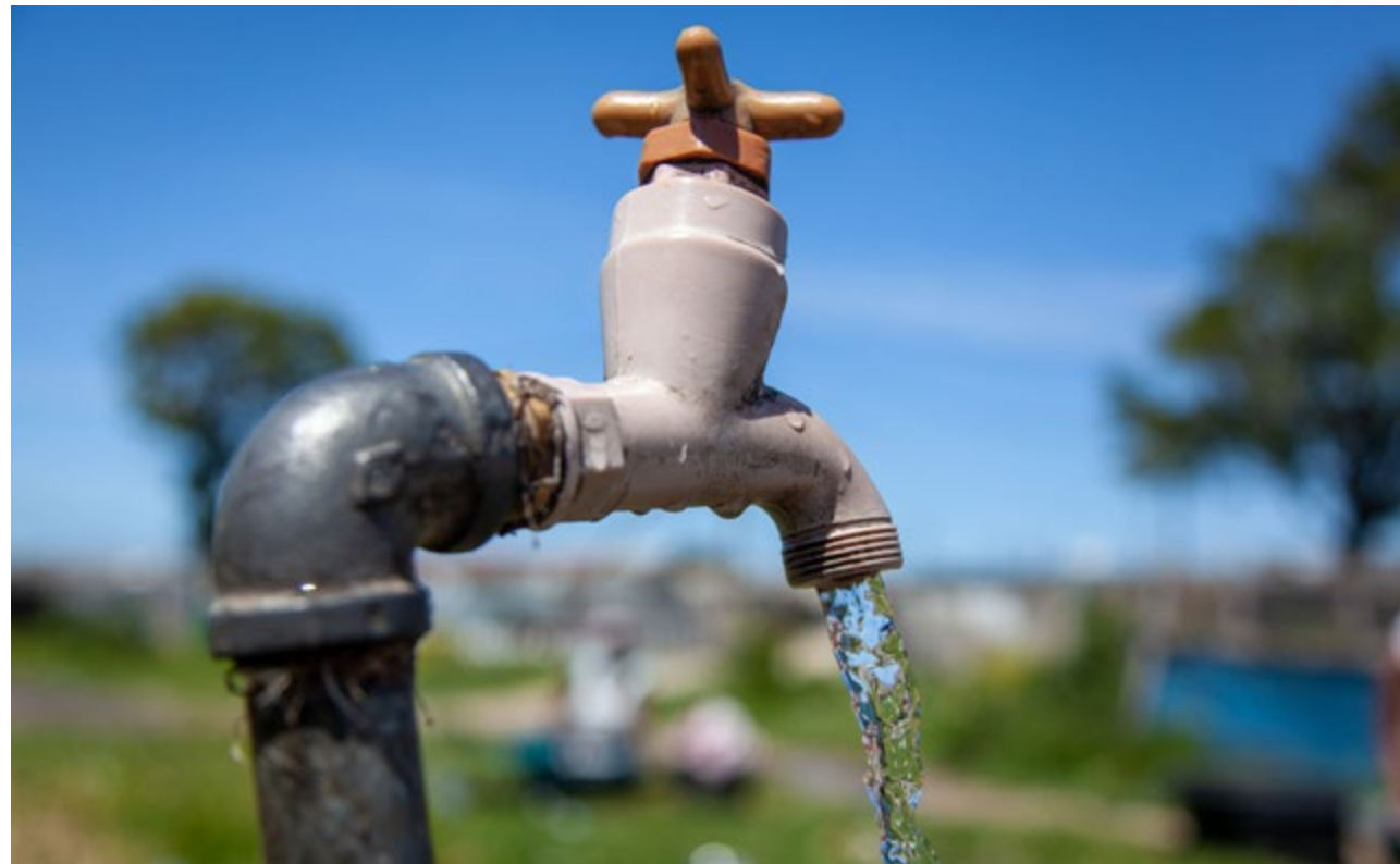
Clean running water should be available and easily accessible to all
